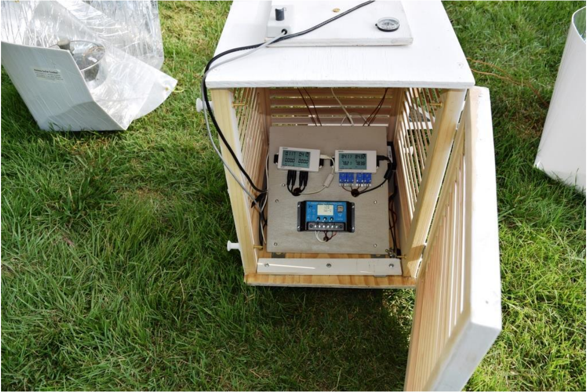
Figure 2 shows the instruments in the interior of the Stevenson box. It contains the two Onset data loggers and a controller for the PV panel. There is a 12V lead-acid storage battery behind the panel.
